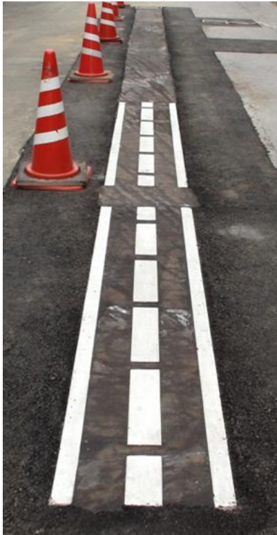
Figure16: Photograph of the constructed test road after paving and lane mark painting
